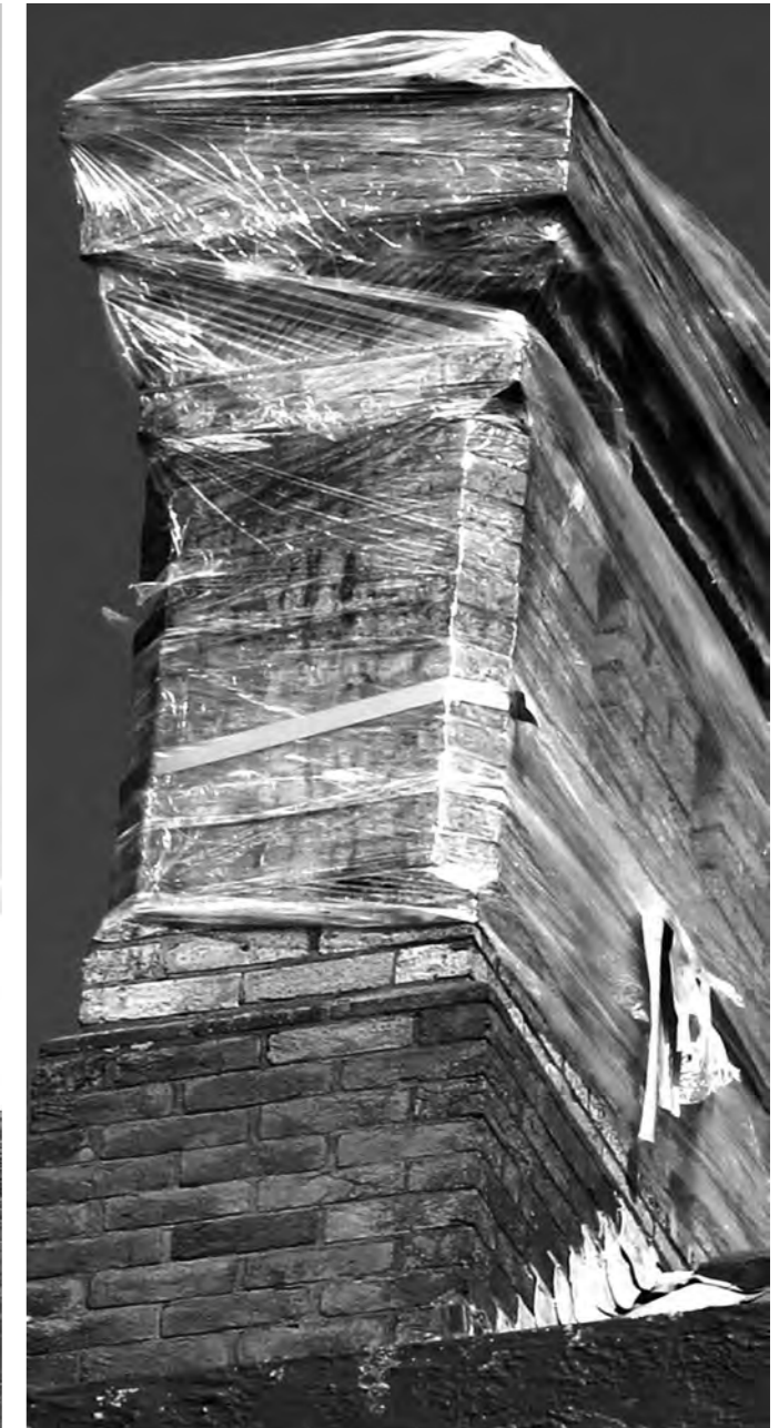
Above left Figure 4: Wrapped chimney, Unitec Institute of Technology, Carrington Road, Mount Albert, Auckland. ©Photo: Author, 2013.
