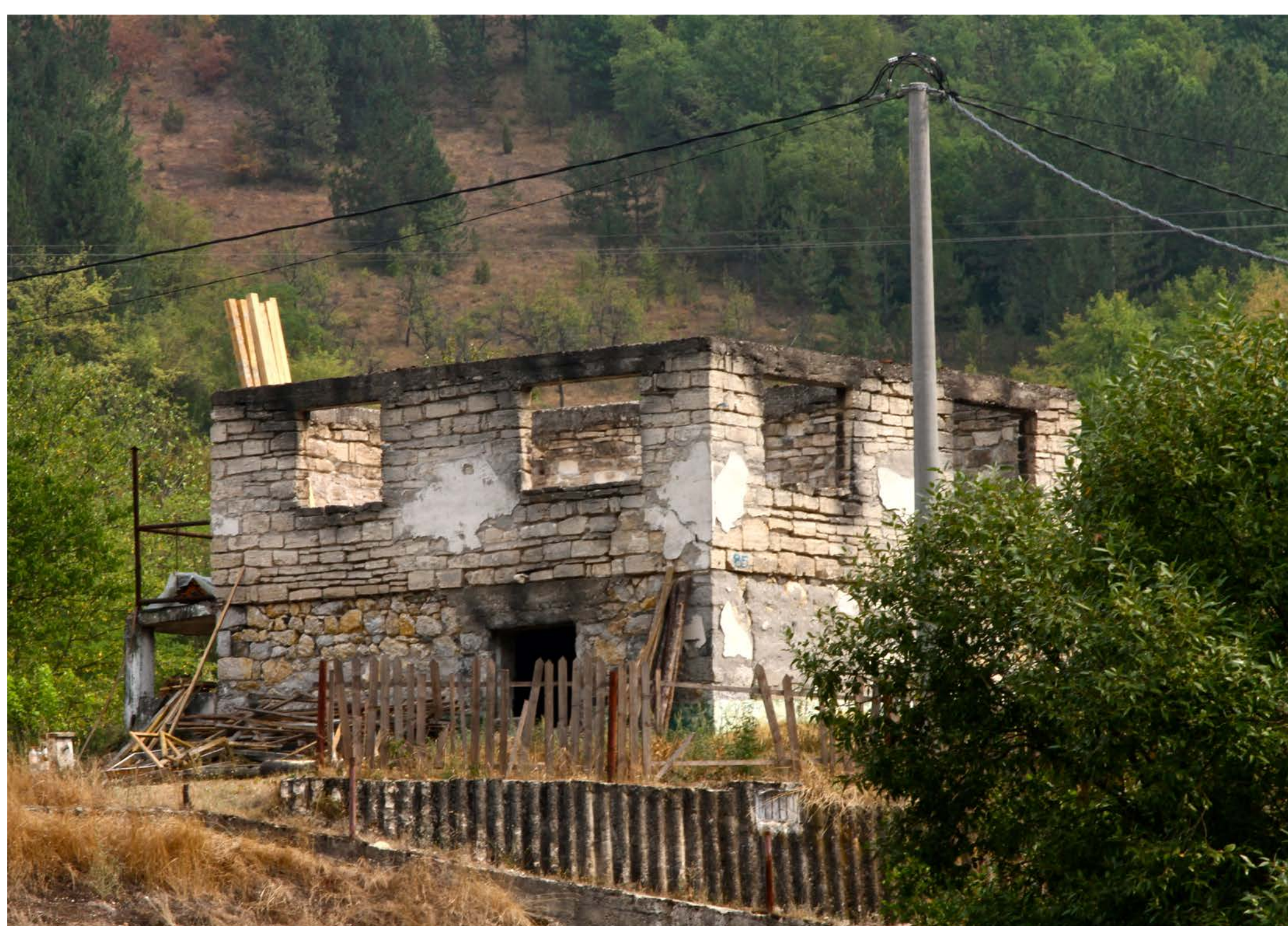
Figure 18. Remaining house structures near the town of Visegrad. Nevena Mrdjenovic, 2012.
