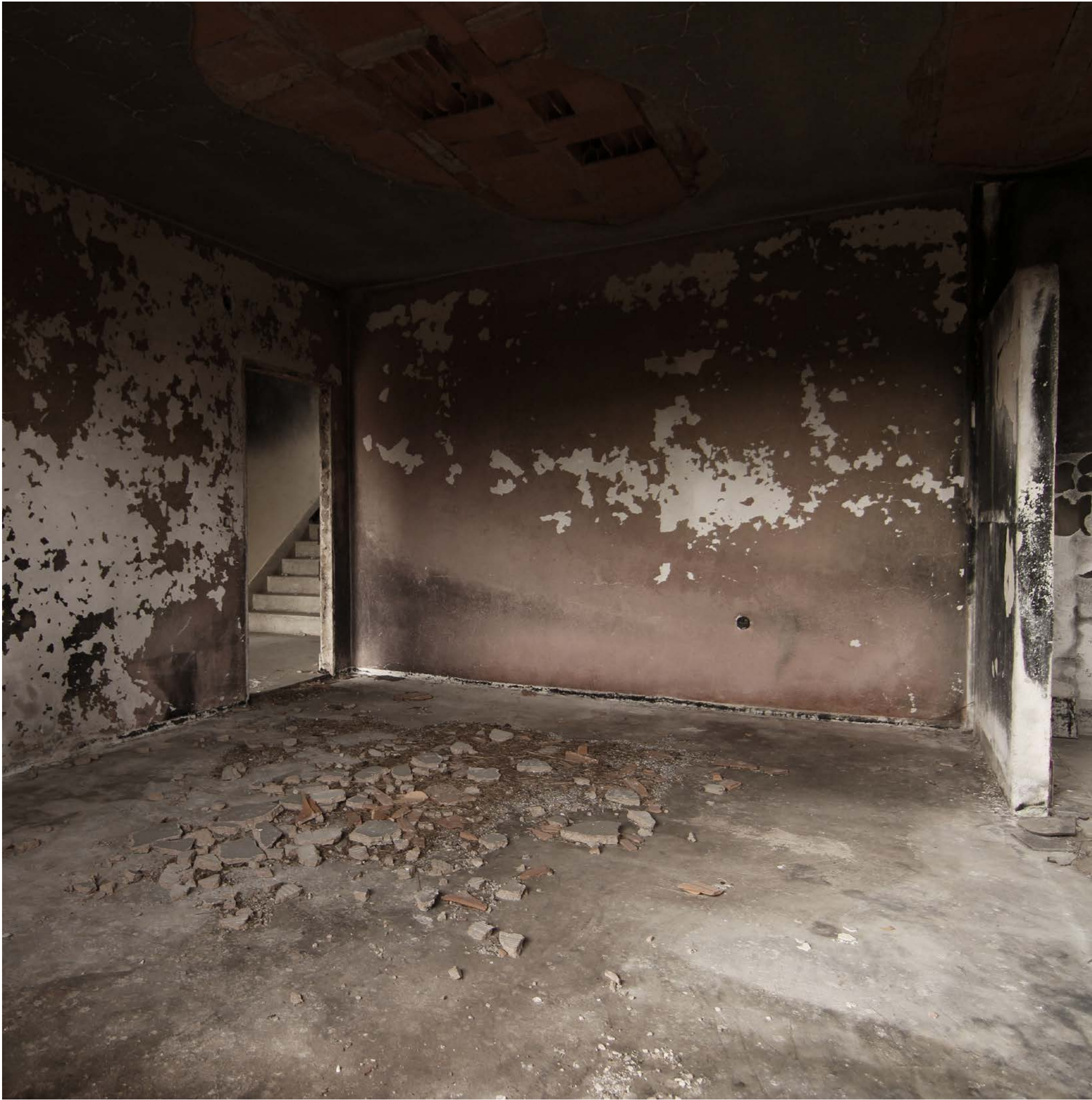
Figure 10. Destroyed interior near the town of Brcko. Nevena Mrdjenovic, 2013.
