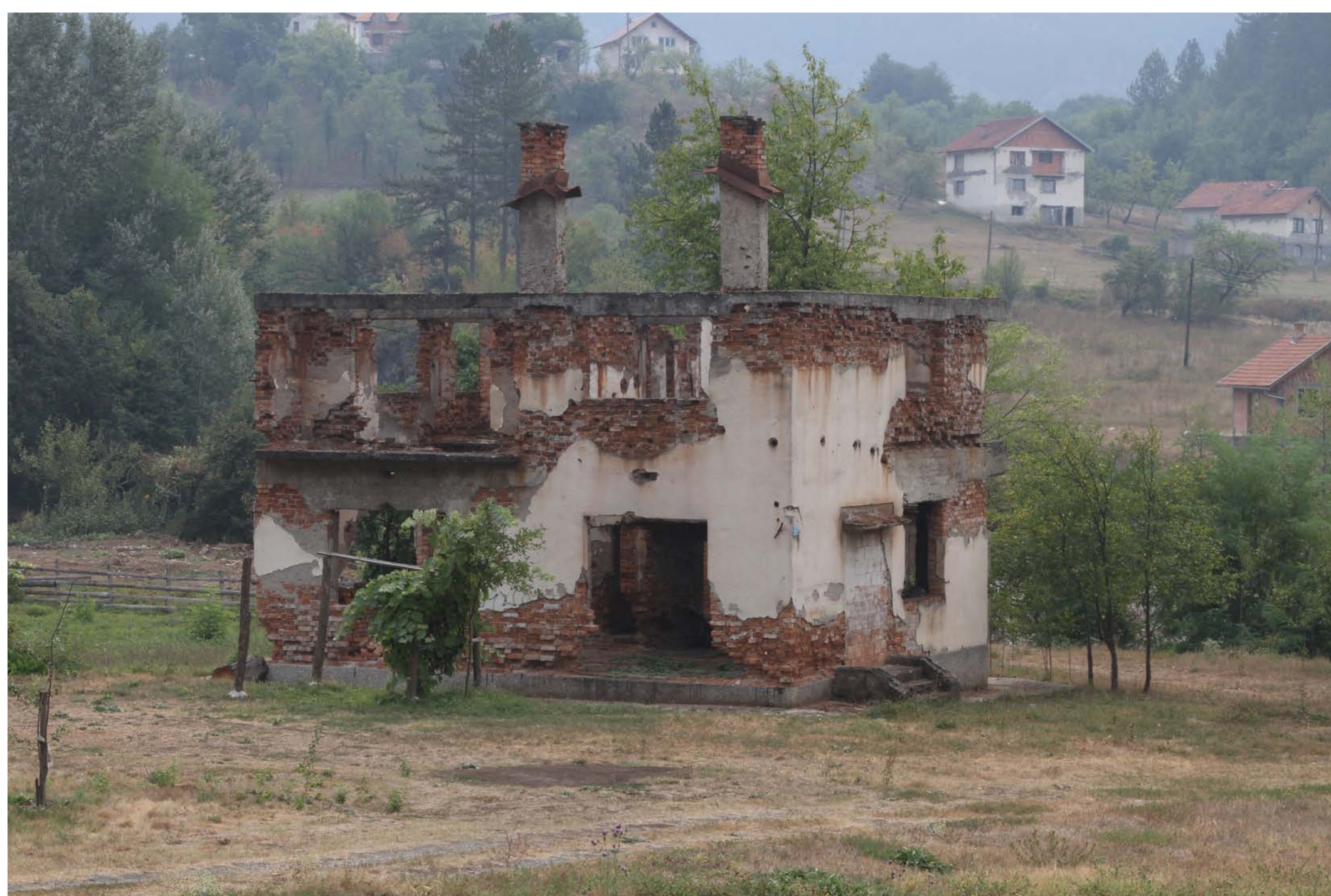
Figure 16. A destroyed house near Visegrad. Nevena Mrdjenovic, 2012.
